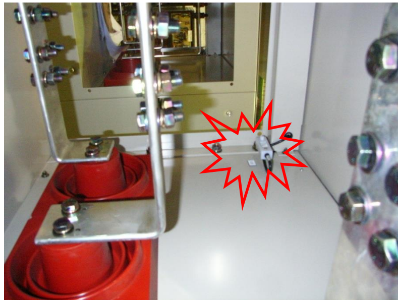
Sensor placement inside busbar chamber
