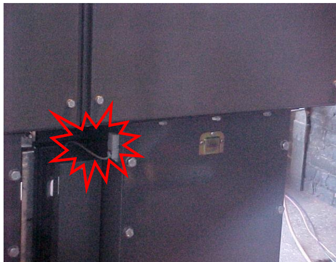
Sensor placement for Switchgear cable termination chamber (External through Hole Detector)
