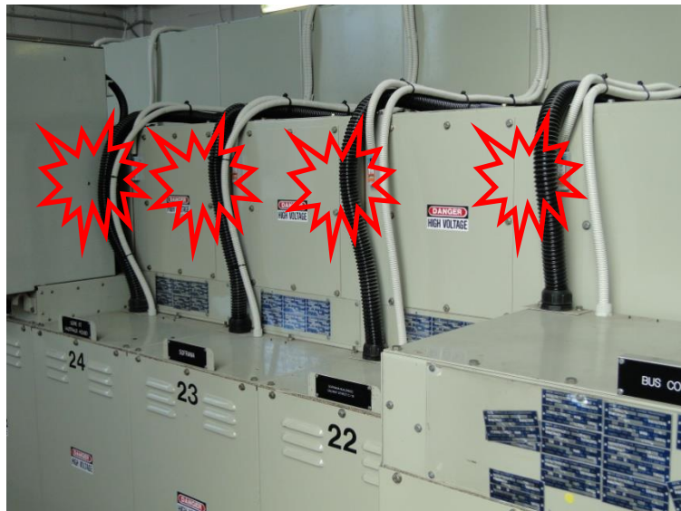
Sensor placement for switchgear Busbar coverage (External through Hole Detector)
