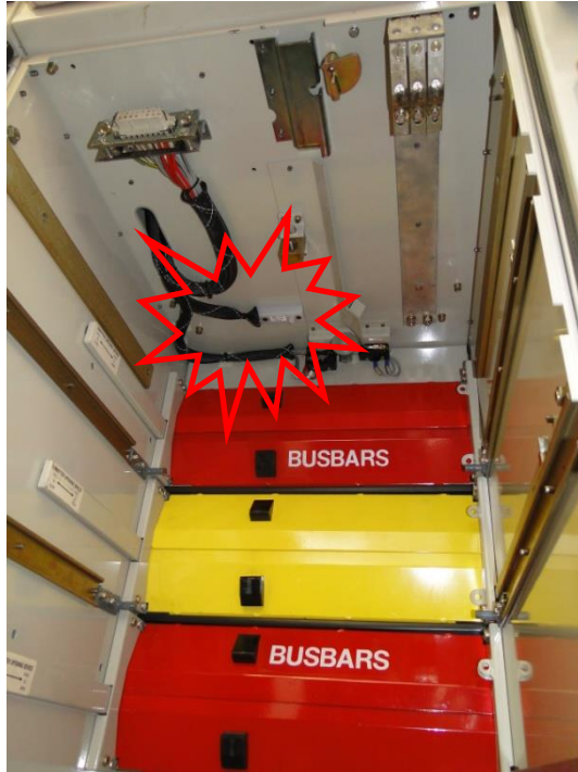
Sensor placement inside CB racking chamber
