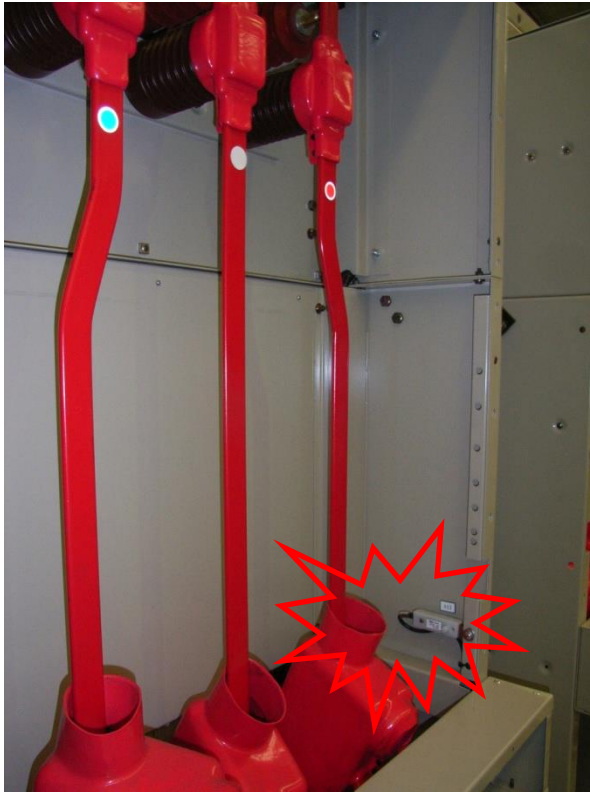
Sensor placement inside cable termination chamber
